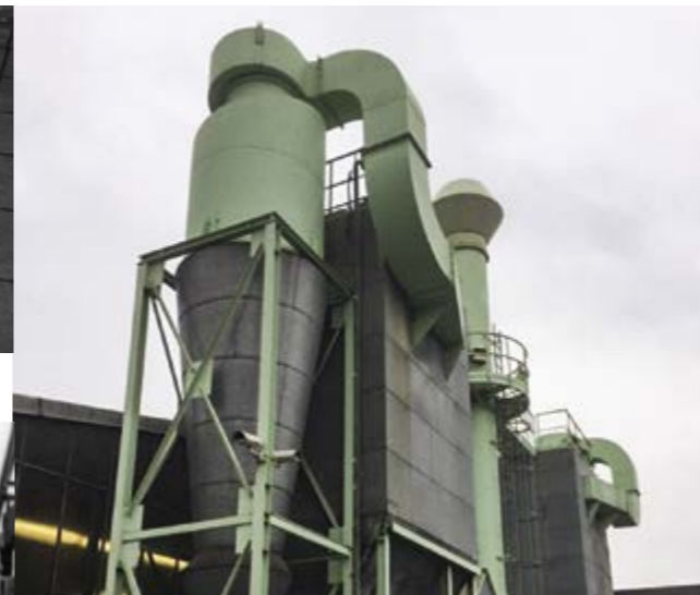
Installation of a modern air filter plant in Andernach
